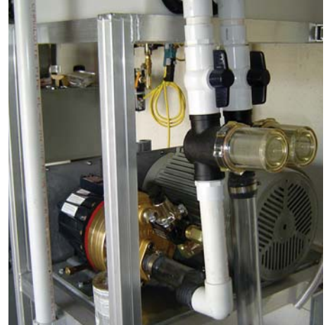
PVC pipe and valves in a car wash application.
