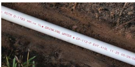
PVC potable water distribution line
