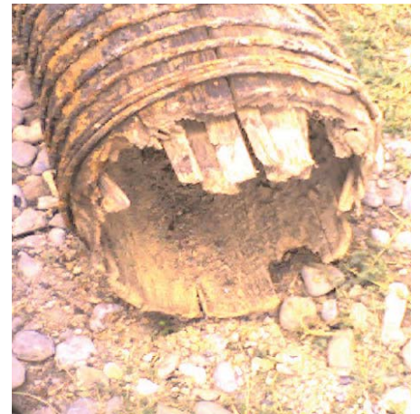
Wood pipe installed decades ago in the New England area of the United States.
