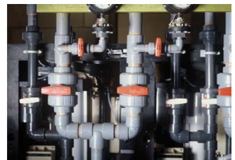
Vinyl valves in chemical processing lines
