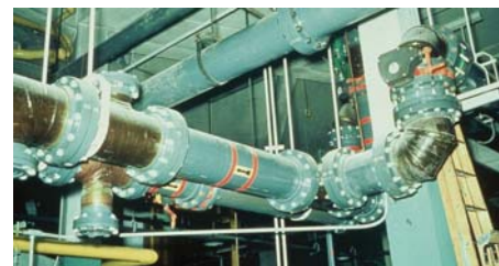
Large diameter PVC piping at Chicago aquarium
