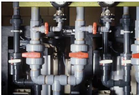
Vinyl valves in chemical processing lines
