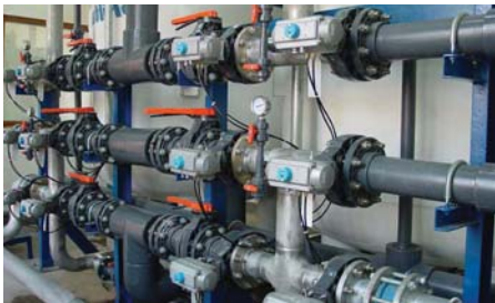
PVC industrial process piping including actuated butterfly valves.
