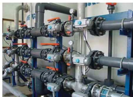
PVC industrial process piping including actuated butterfly valves.
