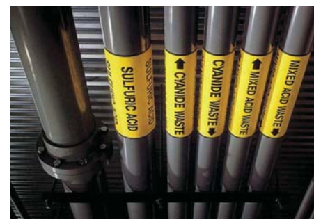
CPVC piping handling chemical process wastes.
